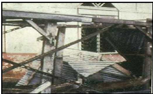
Earthquake damage at Rempi village near Madang
